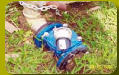
Tubigon, Philippines: Installation of flow meters at all water sources to achieve targets for potable water supply
