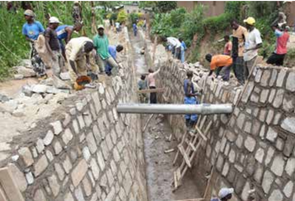
Construction of water tunnel that is supported by UN-Habitat and ONE UN in Bugesera, Rwanda. © UN-Habitat /Julius Mwelu
