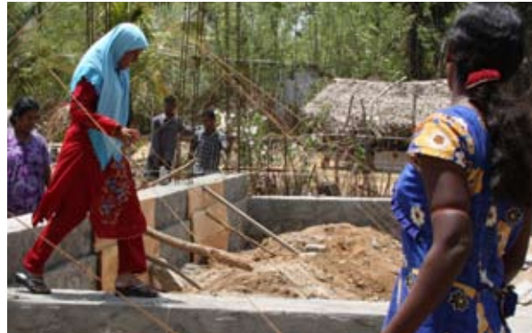
A community in Ampara district works together to build a multipurpose community center
