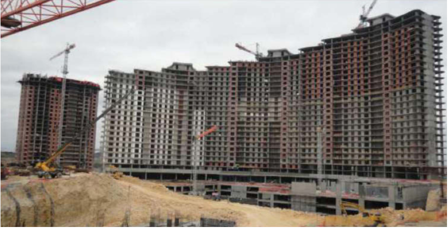
The construction stage of the housing project implemented with a public-private partnership in the renewal area © S.Turk, 2012
