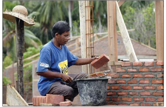
Ensuring the long-term sustainability of shelter is a key challenge for disaster reconstruction
