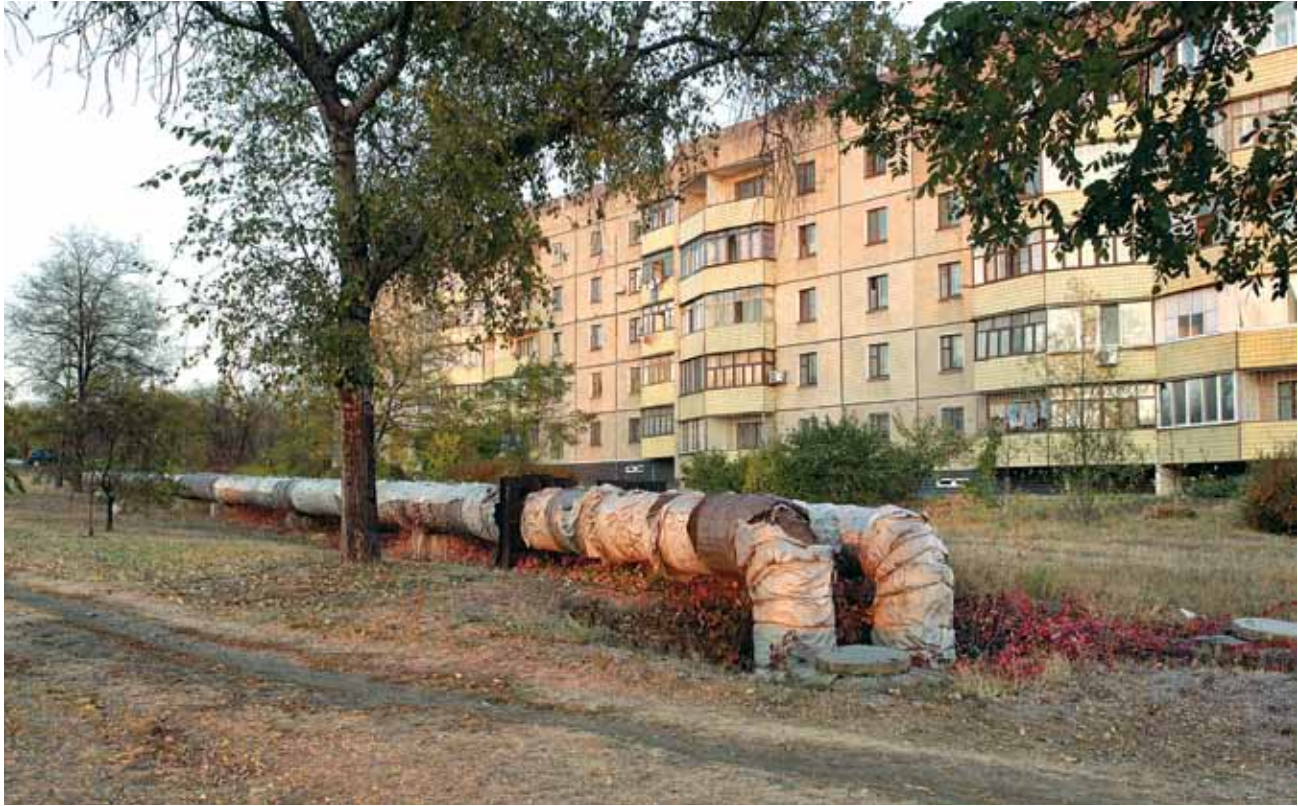
▲ Heating pipes enter the ground next to an apartment block in Krivoy Rog. ©George Georgiou/Panos Pictures
