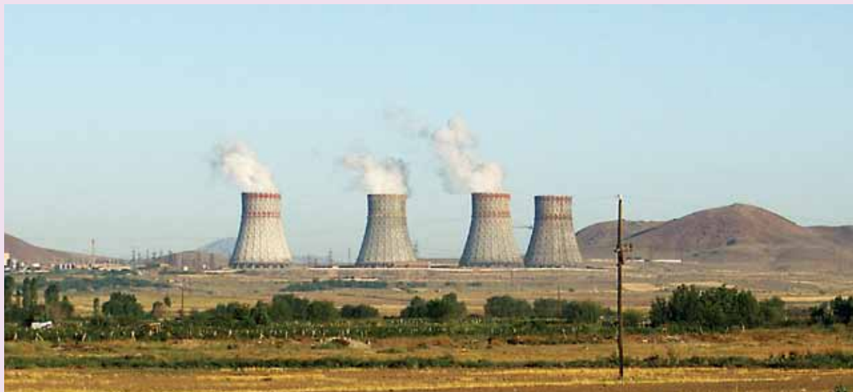
▲ Cooling towers of the Armenian Nuclear Power Plant in Metsamor
