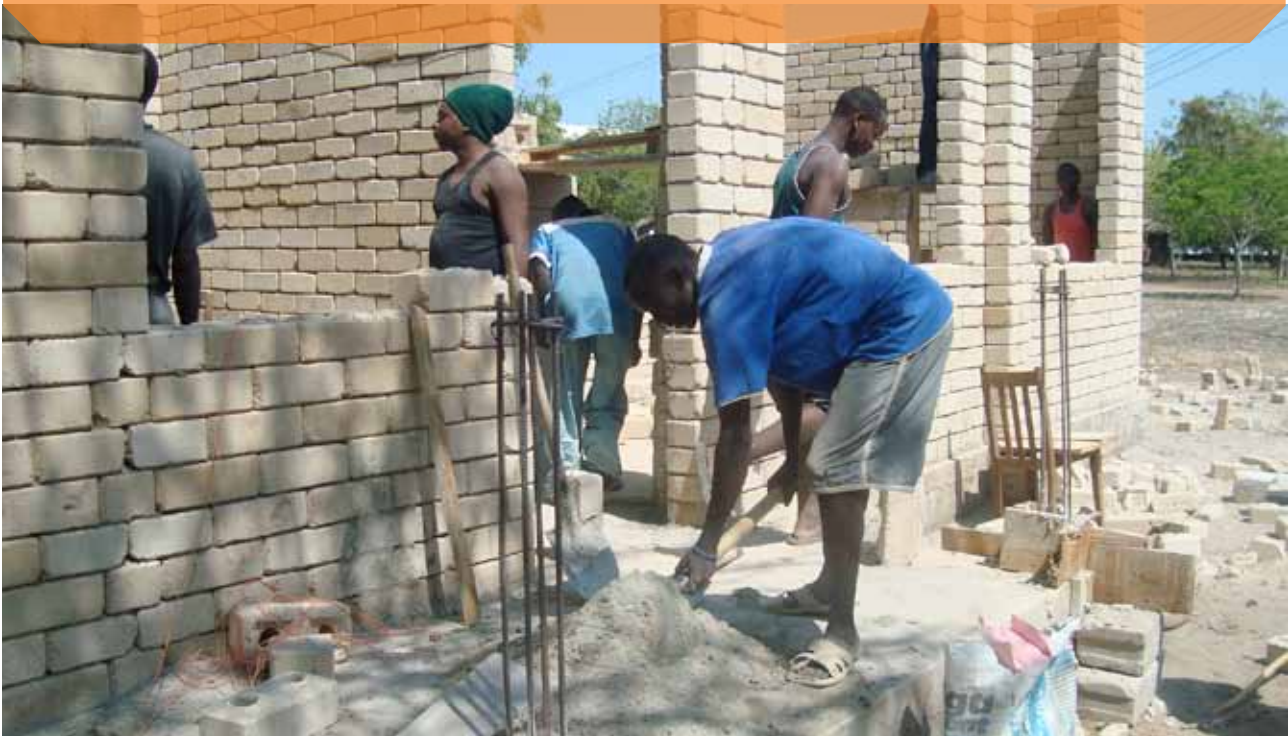
Youth Building Brigades constructing the One Stop Youth Centre in Dar es Salaam. © Gadi Kalugendo
