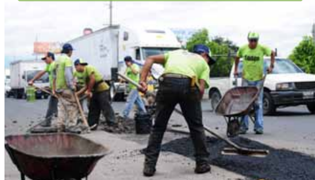
Municipal workers lay asphalt in the Atanasio Tzul avenue, zone 12, Guatemala City, Guatemala. © Maria Fleischmann /World Bank
