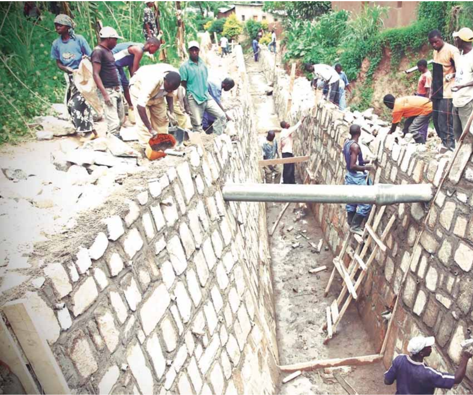
An ongoing construction of water tunnel that is supported by UN-HABITAT and ONE UN in Bugesera, Rwanda 2012 © UN-Habitat /Julius Mwelu
