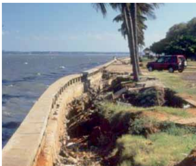
Sea wall to prevent further coastal erosion in Maputo, Mozambique. ©UN-Habitat/Jesper Milner
