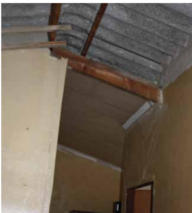
RDP house prior to ceiling installation in Mamre, City of Cape Town, South Africa.
