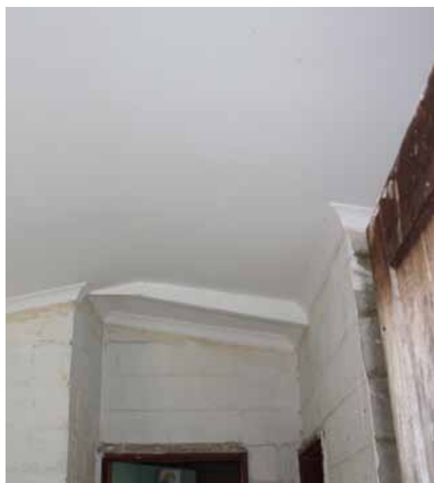
RDP house after 2010 ceiling installation in Mamre, City of Cape Town, South Africa.
