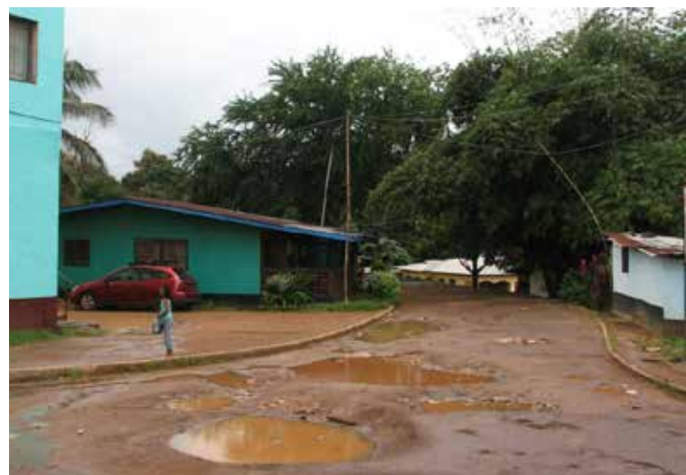
Figure 74. Road in Old Matadi. Note that even metalled roads in government-developed housing areas have little drainage, in one of the wettest countries in the world
