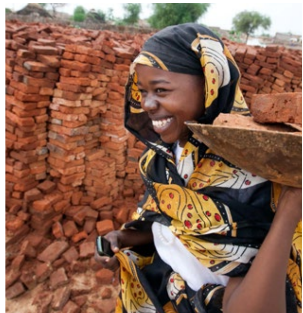
A young woman carries bricks for the construction of a community center in Althoura Shemal in El Fasher, North Darfur. © UNAMID/Albert González Farran
