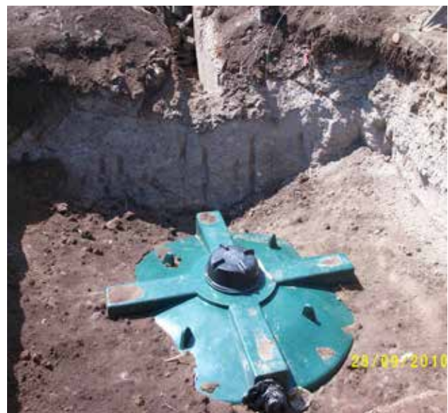
Rotamould tanks used as septic tanks at Koroipita. © SCOPE
