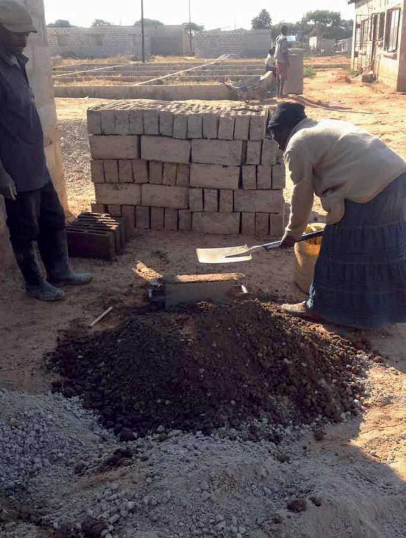
Construction work by community members in an informal area of Lusaka, Zambia © Matthew French/UN-Habitat.
