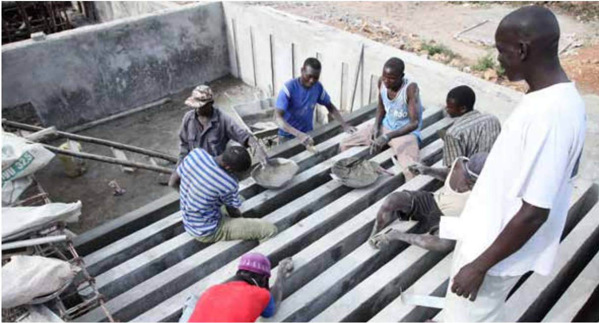
Construction of a new water tank funded by UN-Habitat in Bondo, Kenya, 2011 © UN-Habitat/Julius Mwelu
