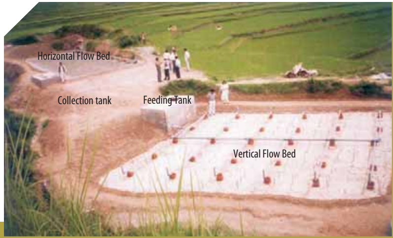
Constructed wetland at Dhulikhel Hospital in 1997 just after the construction (Shrestha R.R., 1999)
