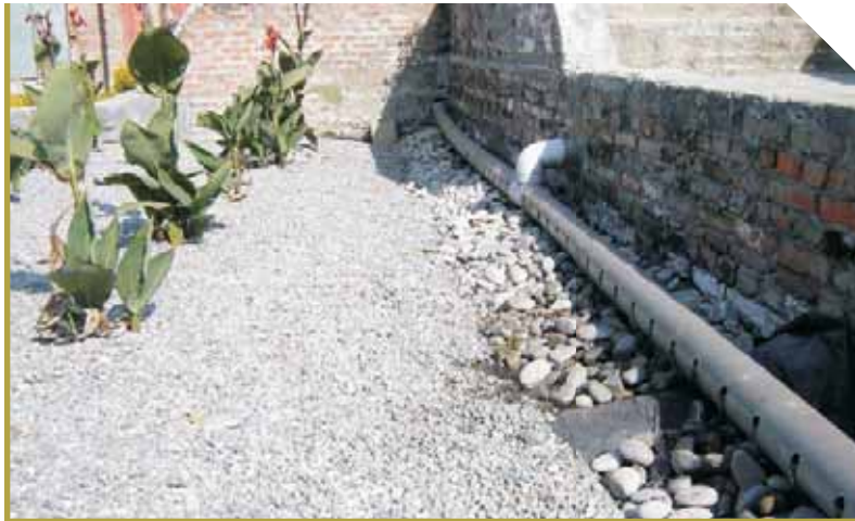
Perforated pipe inlet
