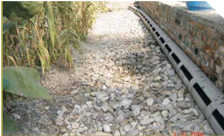
Slotted pipe inlet
