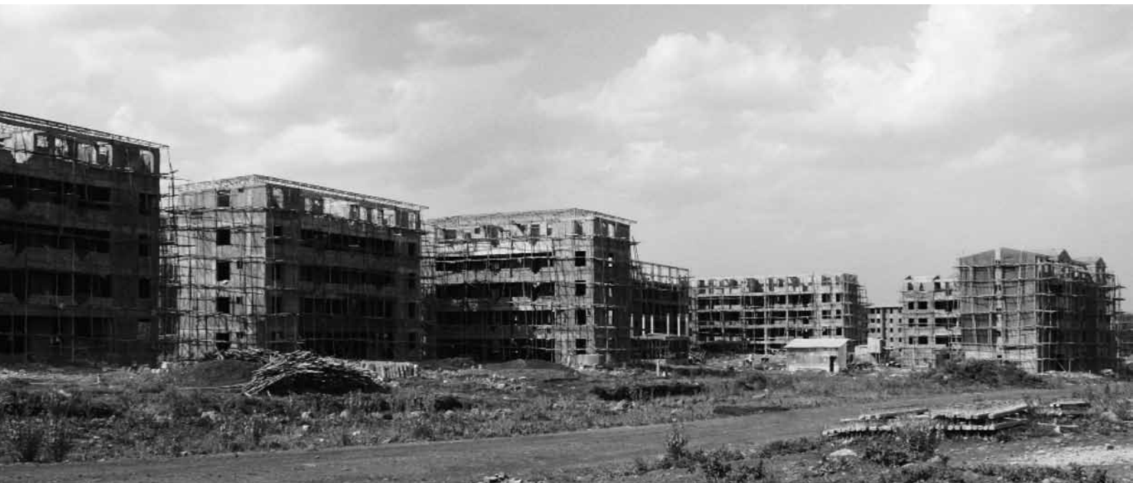
Figure 15: Bole Summit, the last condominium site to be built on the periphery of the city. Addis Ababa. © UN-HABITAT
