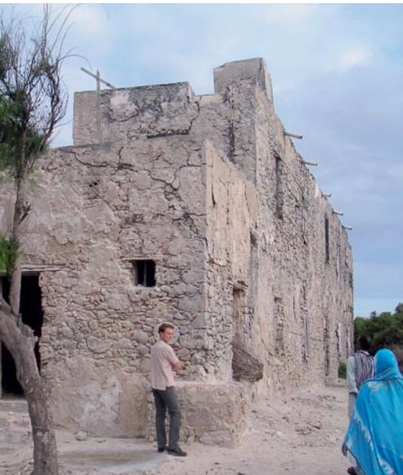
Deteriorated Housing of Swahili architecture in Adaale, Somalia. Photo © UN-HABITAT
