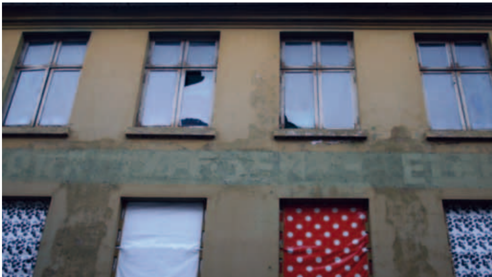
Figure 5: Derelict unused accommodation in Dublin, Ireland. Photo © UN-HABITAT/Matthew French
