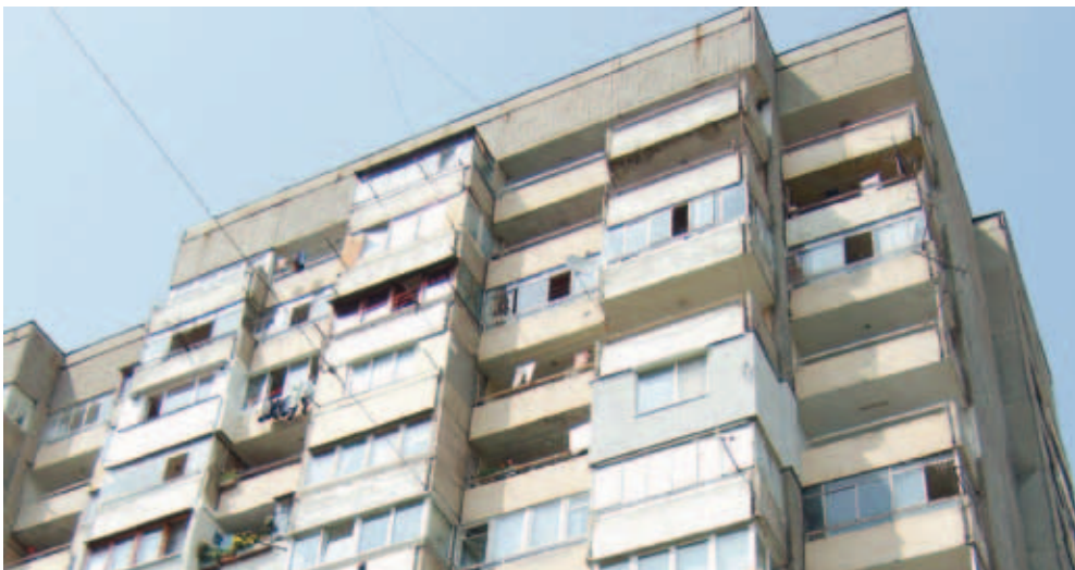
Figure 14: Deteriorated multi-household housing in Bulgaria. Photo © UN-HABITAT/Claudio Acioly
