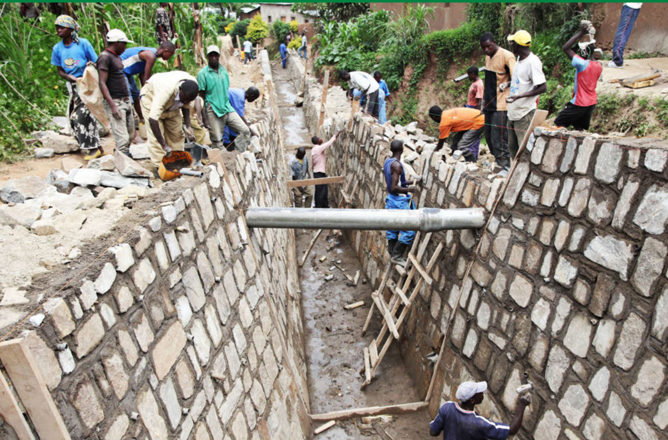
▲ An ongoing construction of water tunnel supported by UN-HABITAT and ONE UN in Bugesera, Rwanda 2012. © UN-Habitat/Julius Mwelu
