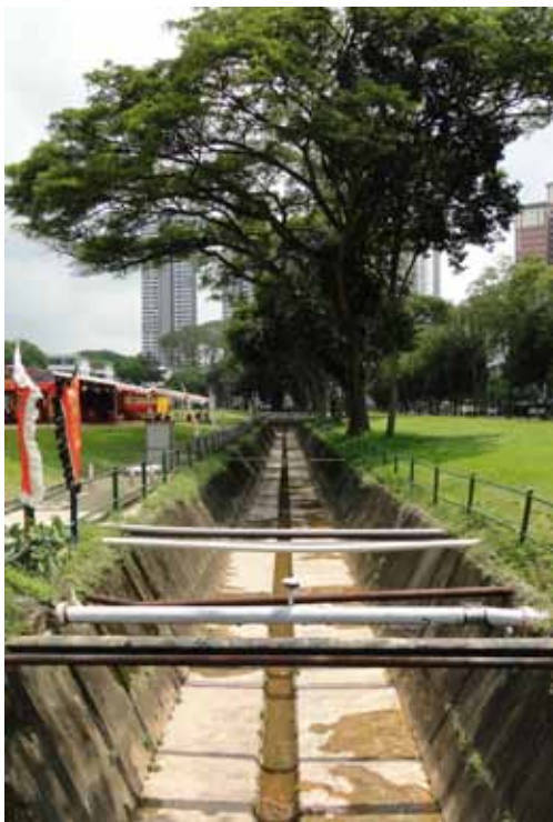
Storm water collection infrastructure is integrated into public green space © UN Habitat/Andrew Rudd
