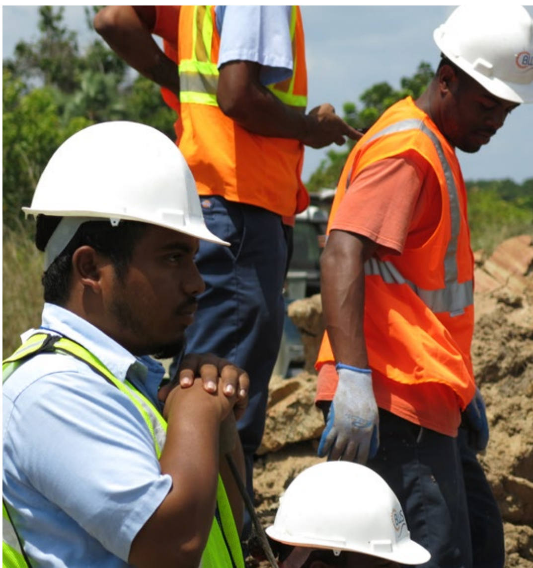
WOP between BWS, Belize & CCWD, California - BWS employees at work, repairing a leak on the main to Belize City.
