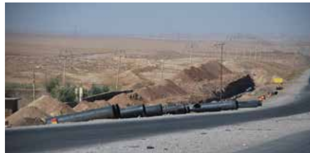
Excavation work in the Right Bank Water project before ISIL © UN-Habitat / Iraqi Urban Observatory
