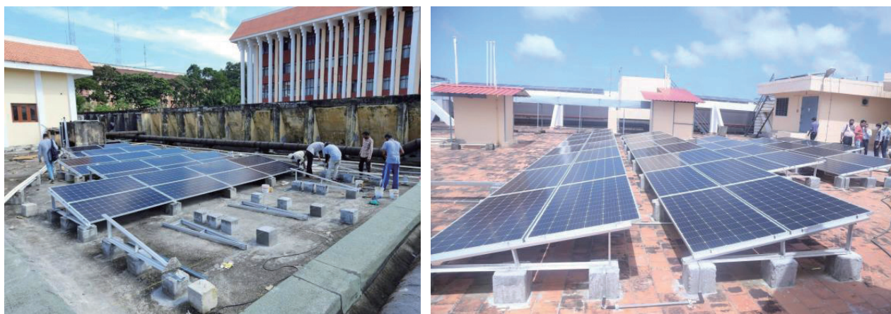
Figure 2.41 Solar installations on government buildings' rooftops
