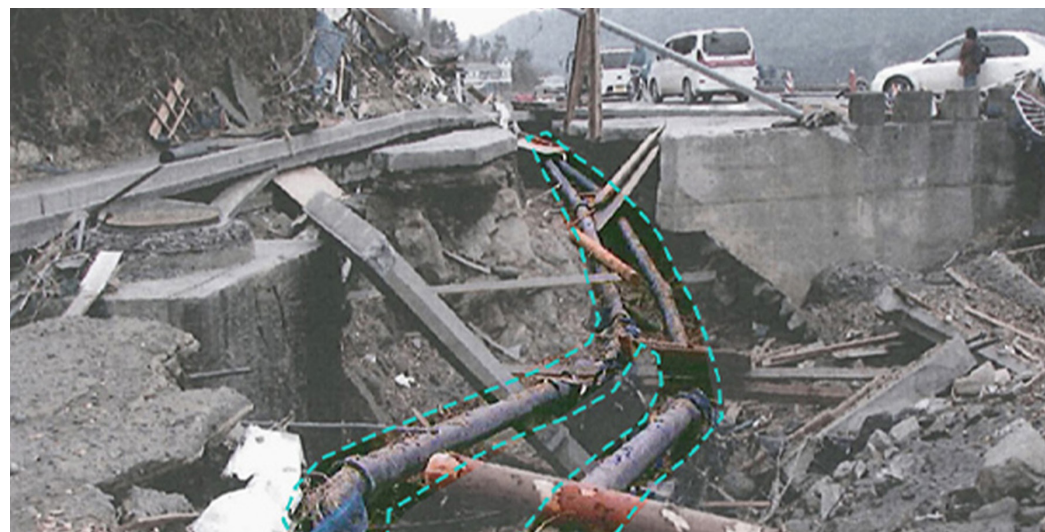
Fig 27. Earthquake-resistant ductile iron pipes exposed after the 2011 Earthquake in Japan
