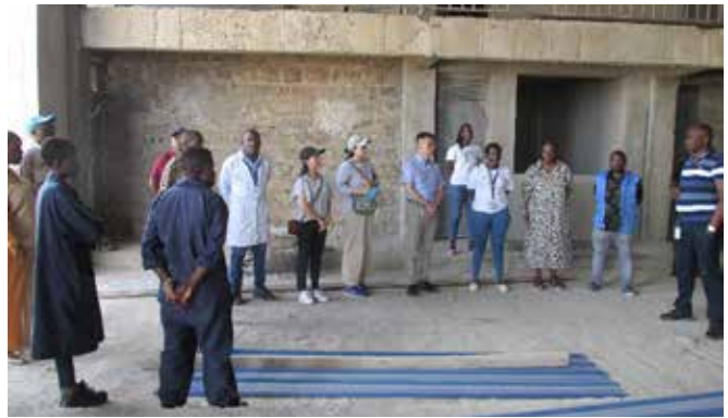
At the UN Women Garage project which is under construction. The Garage supported by Toyota will provide equal access to women to get technical skills. © UN-Habitat
