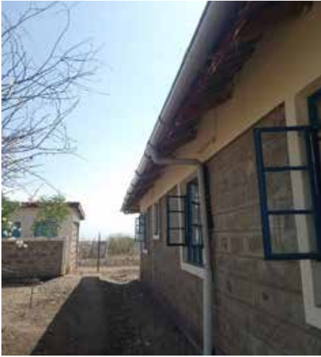
Top left: Rainwater collection gutters and downpipes. © UN-Habitat
