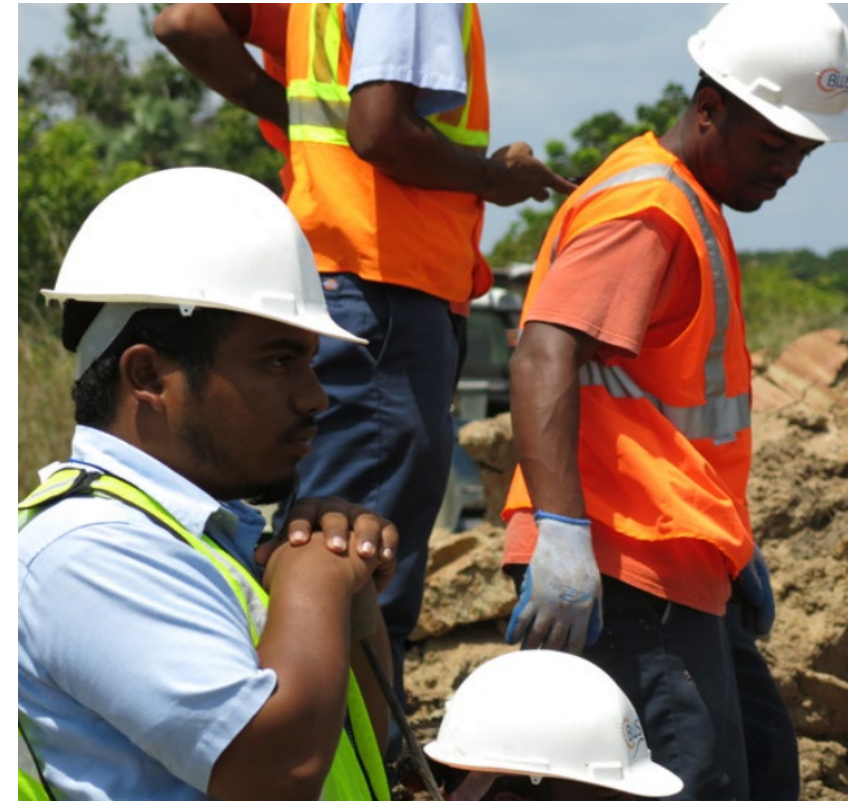
FIGURE 4. BWS EMPLOYEES AT WORK, REPAIRING A LEAK ON THE MAIN TO BELIZE CITY © VINCENT MERME / GWOPA-UN-HABITA
