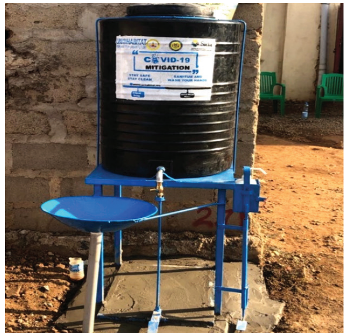
Figure 52: Installed handwashing station in Juba
