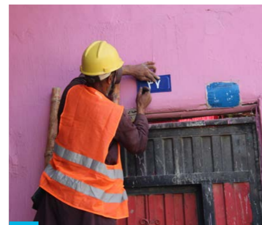
As part of the programme to regularize urban informal settlements, a worker installs a house number above a door in Kabul © UN-Habitat/Afghanistan
