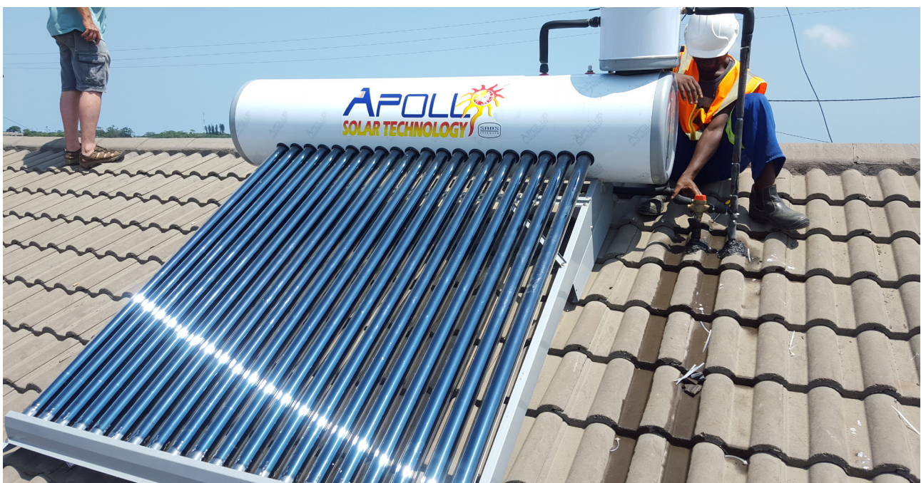
Solar water heaters installed in KwaDukuza, South Africa during Phase 1. © UN-Habitat
