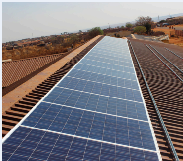
Solar panels are installed on a community centre in Steve Tshwere Local Municipality, South Africa, during phase I of the Urban-LEDS project.
