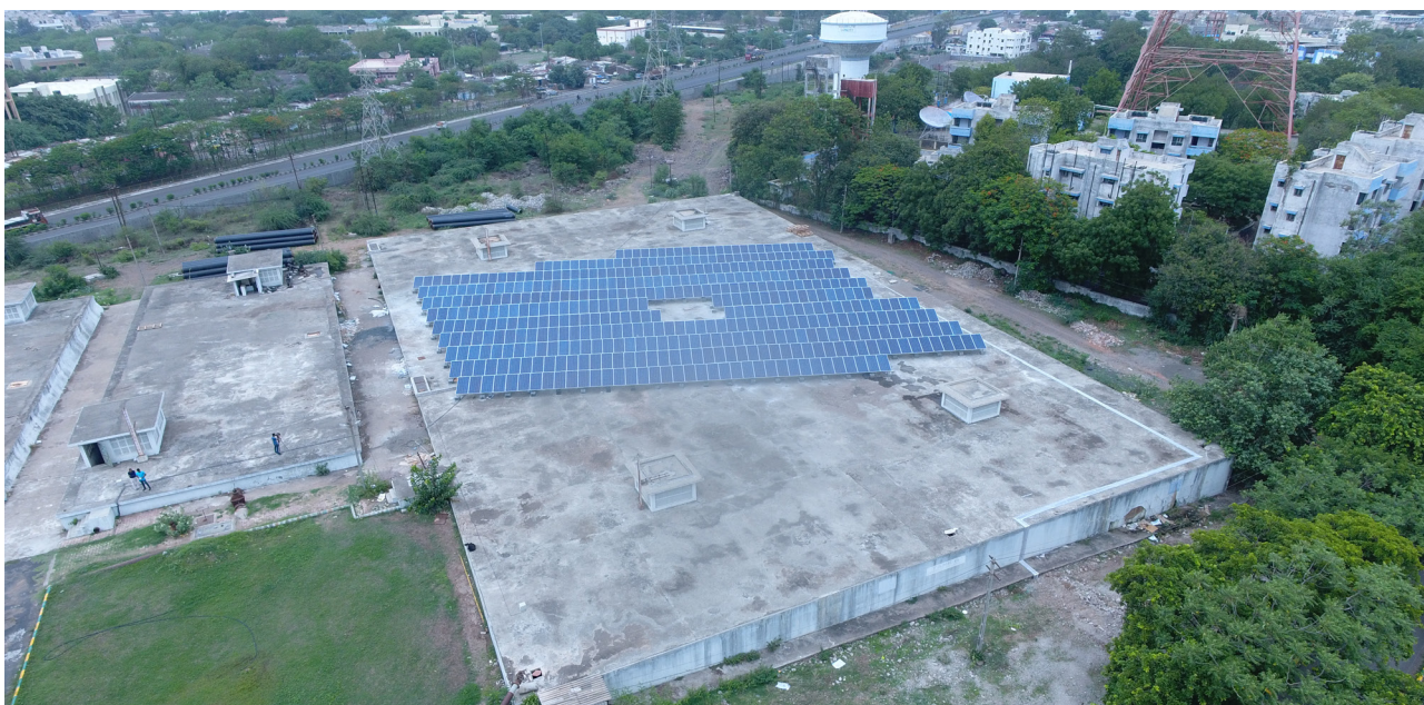
145-kilowatt solar PV system installed at the Aji Water Treatment Plant, Rajkot © Rajkot Municipal Corporation
