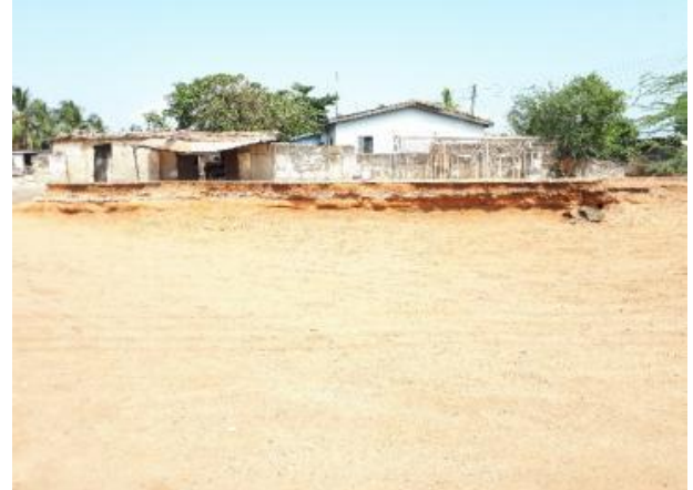
Figure 5.10: Coastal Erosion at Vodza
