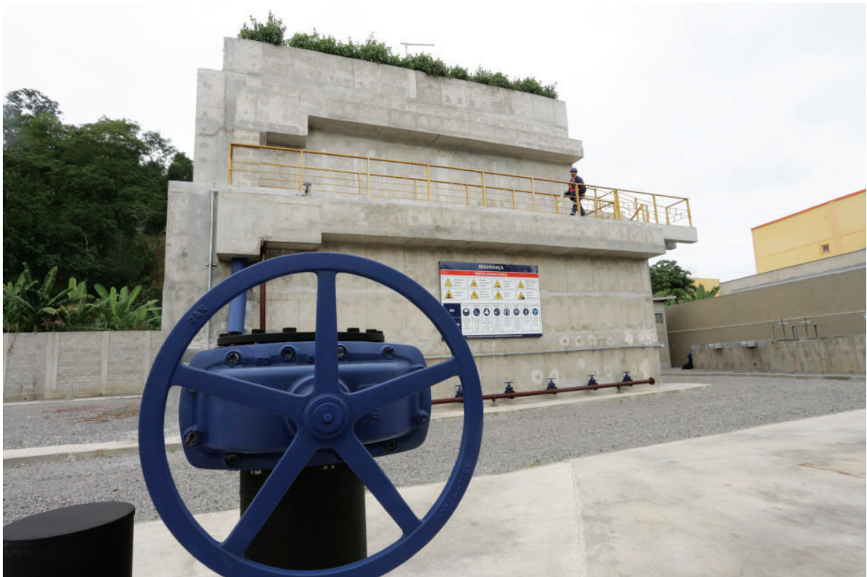
Sewage Treatment Plant (ETE) Maria Paula.
