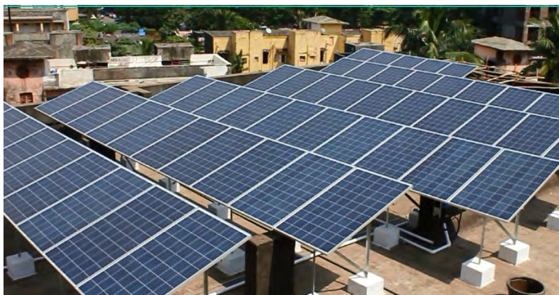
Solar PV System at municipal school in Thane ©ICLEI South Asia
