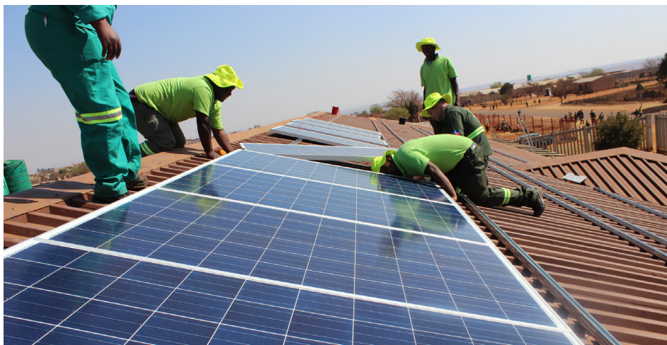
Solar PV installation at a community centre in South Africa during phase 1 of the project. © Grace Stead
