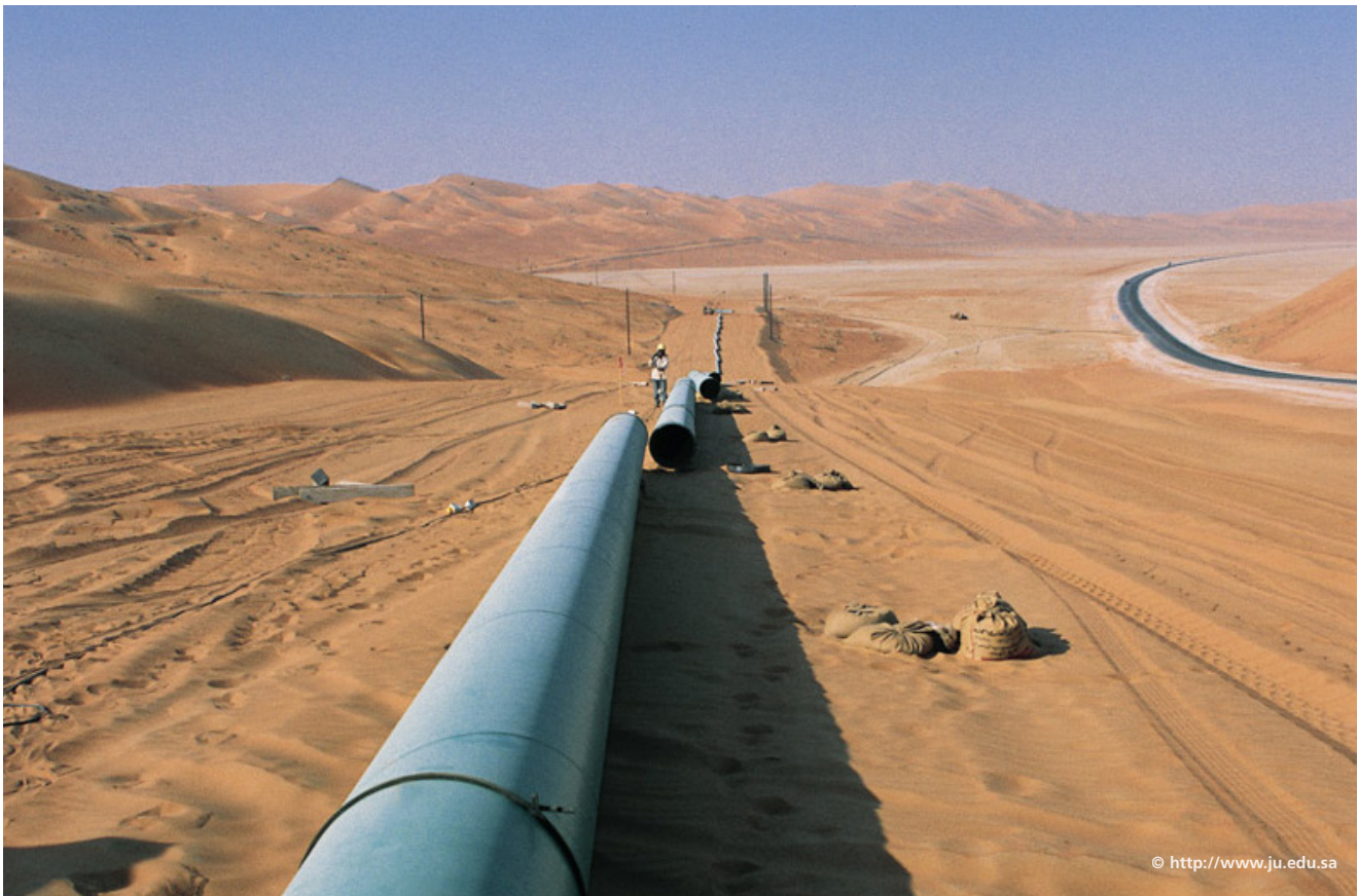
Oil pipelines along the territory of the Eastern Region
