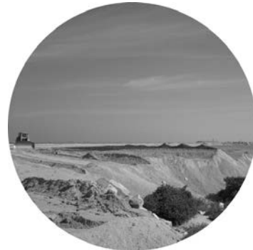
Land reclamation is one of the most disruptive activities to coastal and marine resources.
