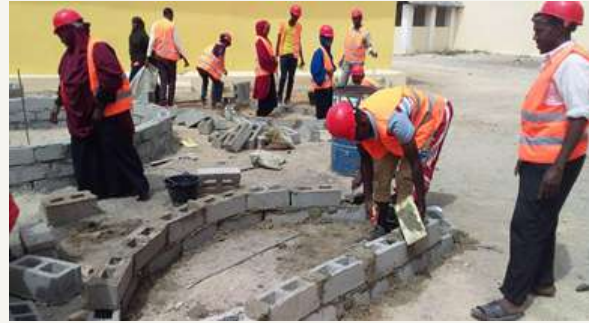
Youth practising new construction skills at the Banadir University training centre, Jubaland, Somalia © UN-Habitat.
