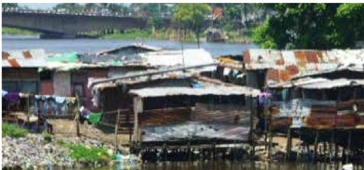
A dilapidated settlement with poor structural integrity
