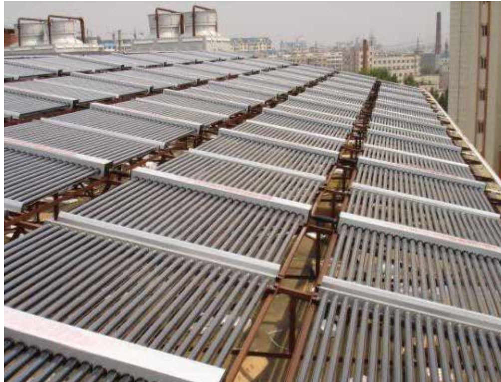
Image: Industrial system solar water heater. © UN-Habitat
